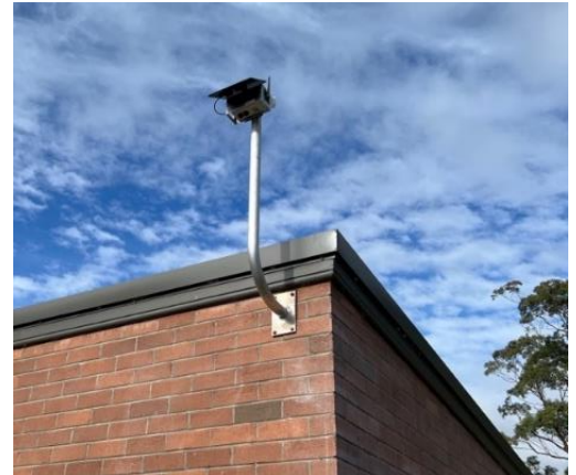
A J-pole extension installed in Sutherland Shire (NSW) for the purpose of mounting a Clarity air quality sensing device.
