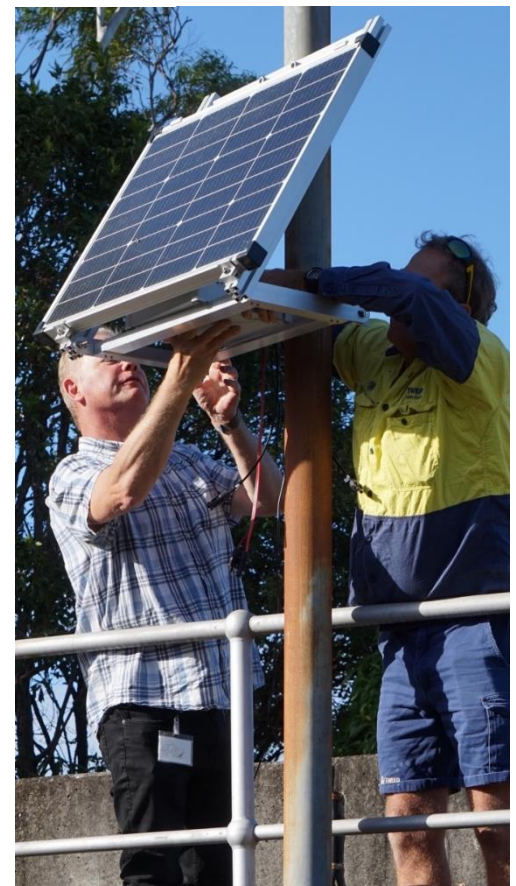
Installation of an air quality sensing device and solar panel in Tweed Heads, NSW. Image source: Tweed Shire Council
