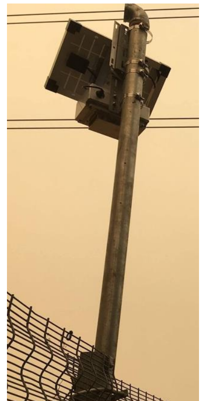
Heavy bushfire smoke in Parramatta, NSW. Smoke can attenuate wireless signal strength, resulting in lost communications. Image source: UTS.
