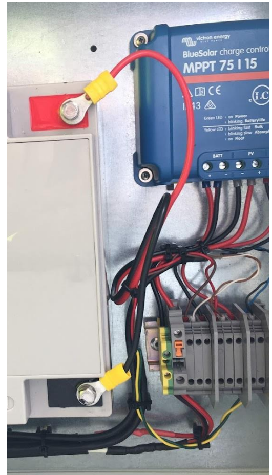
A battery should ideally be integrated with a charge controller that prevents 'depth of discharge' (DoD) exceedances, avoiding permanent battery damage. Image source: UTS.
