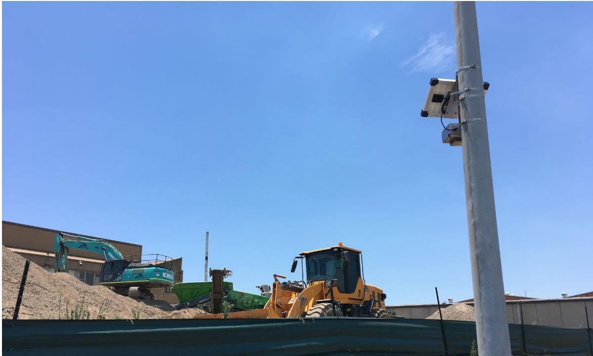
A low-cost particulate sensing device installed to monitor dust arising at the construction site, Parramatta, NSW. Image source: UTS
