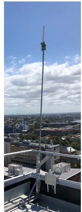
A LoRaWAN gateway on a rooftop in Sydney, Australia. Image source: UTS
