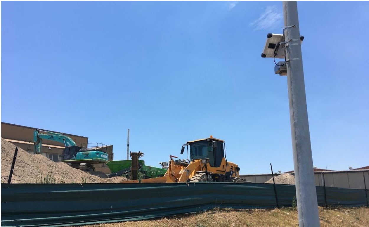
Sensing devices installed to monitor dust at a construction site in Parramatta, NSW. Image source: UTS
