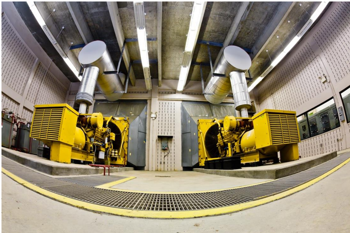
Most commercial buildings have at least one backup generator in their basement, and larger buildings may have several.
