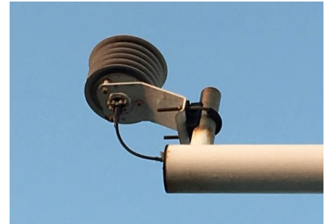
A temperature and humidity sensing device deployed on an ocean pier, suffering from rust corrosion. Image source: UTS
